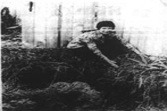
City water repair problem
