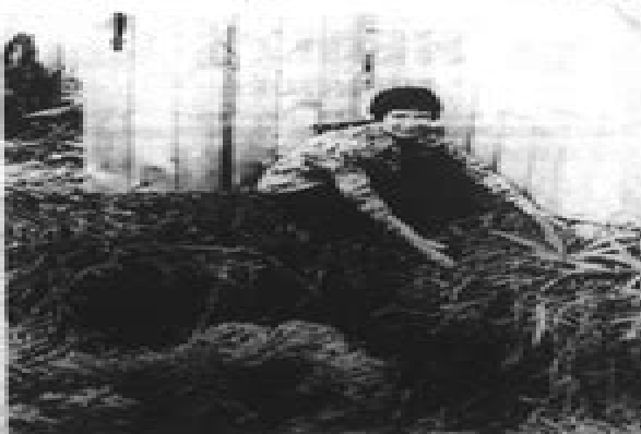
City water repair problem
