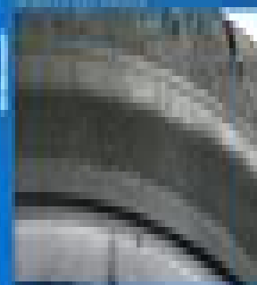
Excessive Sidewall Abrasion
